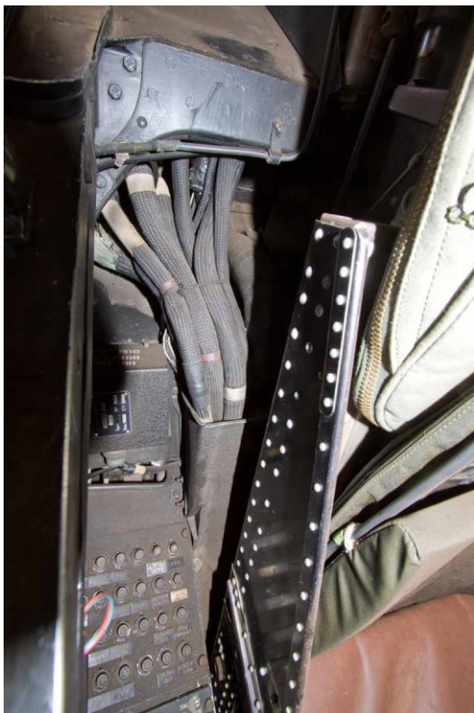
Cluttered rear right hand bulkhead with electrical harness lines and what appears to be a fuse panel.
